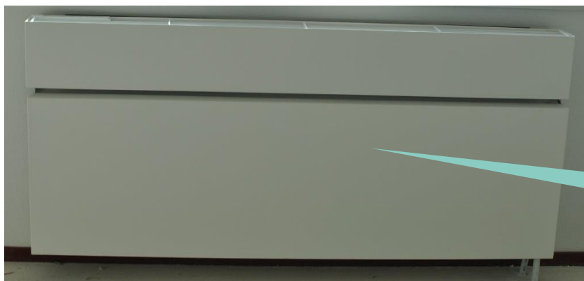
Horizontale radiator in woonkamer/studio
